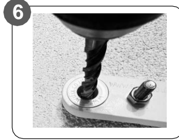
6 Drill through tube into substrate to the appropriate depth for fixing (site specific).
